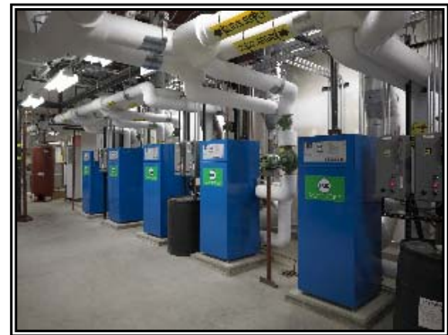
Figure XII: Hot Water and Glycol Boiler Systems
